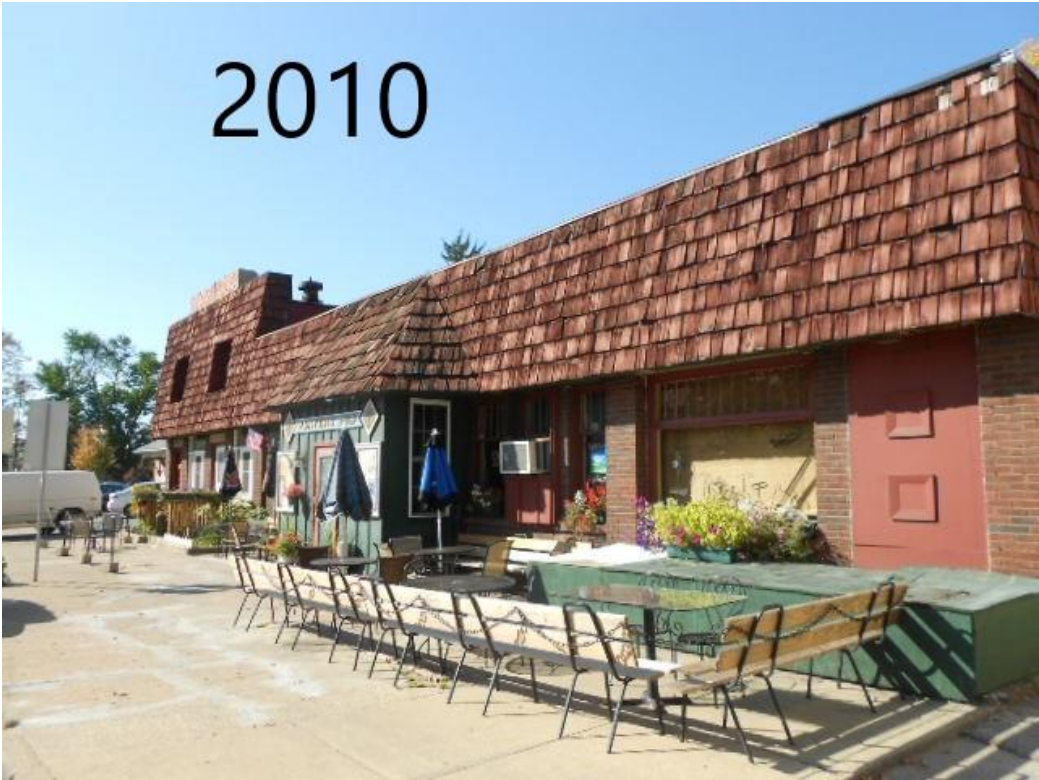
Photo taken in 2010 shows that the lower half of the façade has been restored and windows opened.
