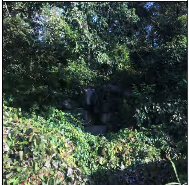
Photo 8: Limestone blocks in sinkhole area on northeastern portion of Site; View to the north
